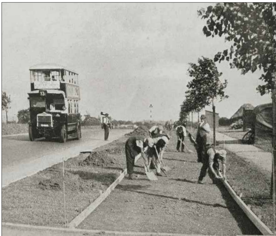
Figure 2. Work in progress on construction of a 1930s cycle path in London. The designated path is being dug out in preparation for filling with concrete to form a solid smooth surface.
